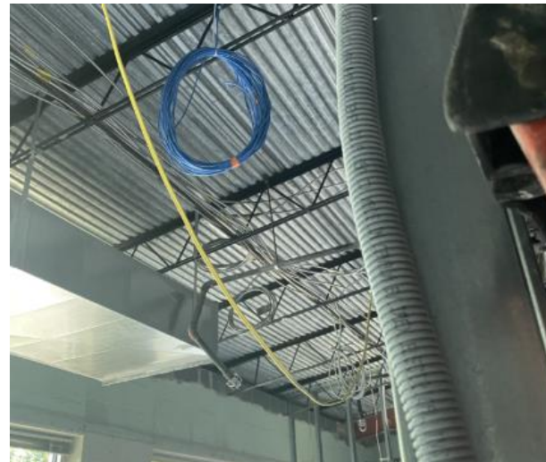
Low Voltage lines in Kitchen
